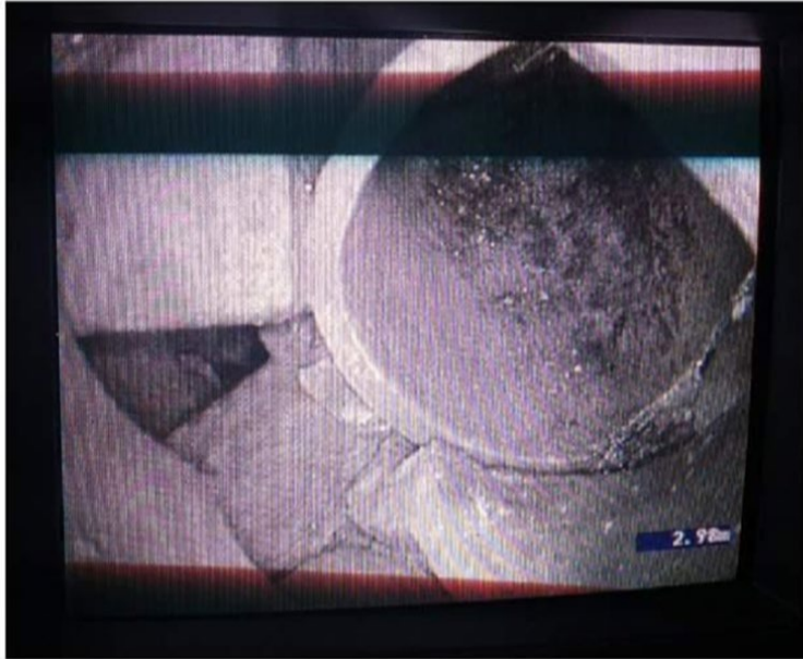
Defective lateral connection prior to 2K Injection repair
