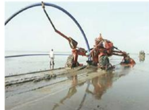
Open trench not possible, but with pipe plough in wet fields it works!
