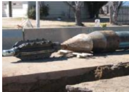
Crack brittle pipes: clay, asbestos, cast iron, PVC
