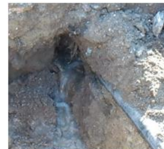
PE40 pipe damage
